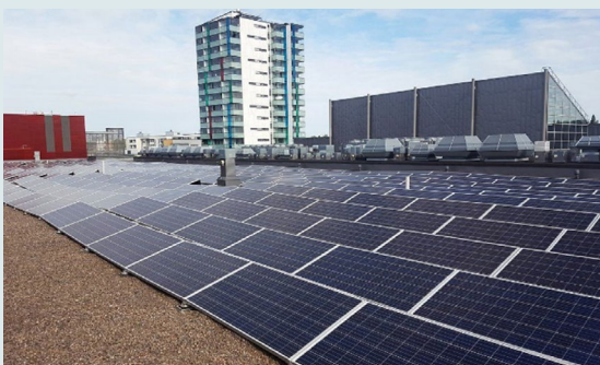
Figure 5.5 - The shopping centre Sello has a photovoltaic plant with a total power of 550 kWp. Batteries can take the load if over production occurs.
